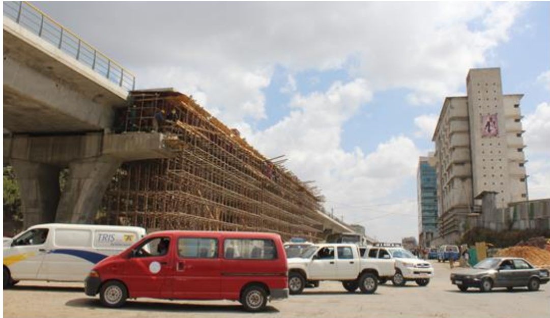
Addis Ababa Light Rail Tram under construction December 2014. Photo by Donielle DeToy
